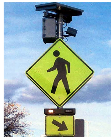
Top: Fiberglass pre-fabricated bridge Middle: LED trail lighting Bottom: Solar-Powered LED Pedestrian Crossing Warning/ Flashing Sign
