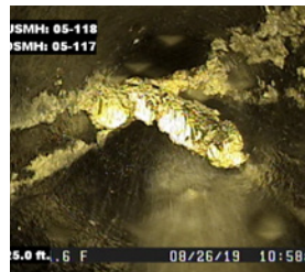
Private lateral and City sewer pipes clogged due to grease.
